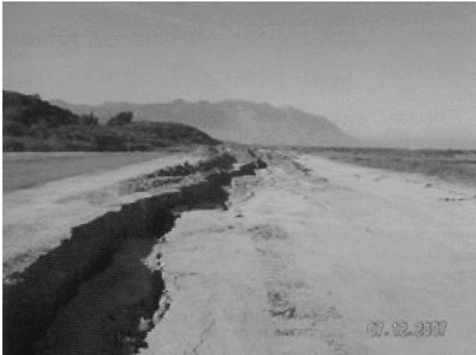
Crack and settlement (Athens-Thessaloniki highway)
