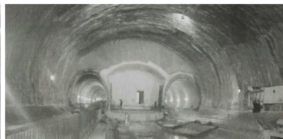
Aegaleo station cavern
