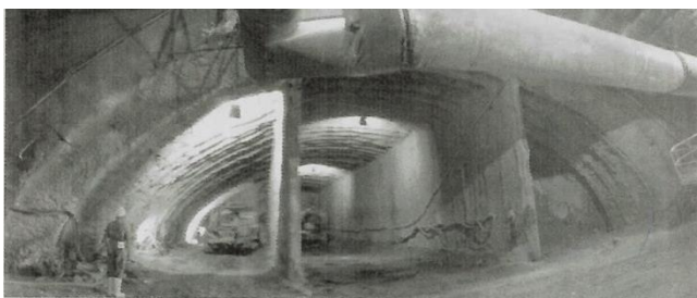
Aegaleo station cavern
