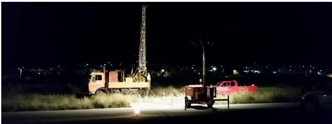
Drilling rig working at night next to the airport take off corridor
