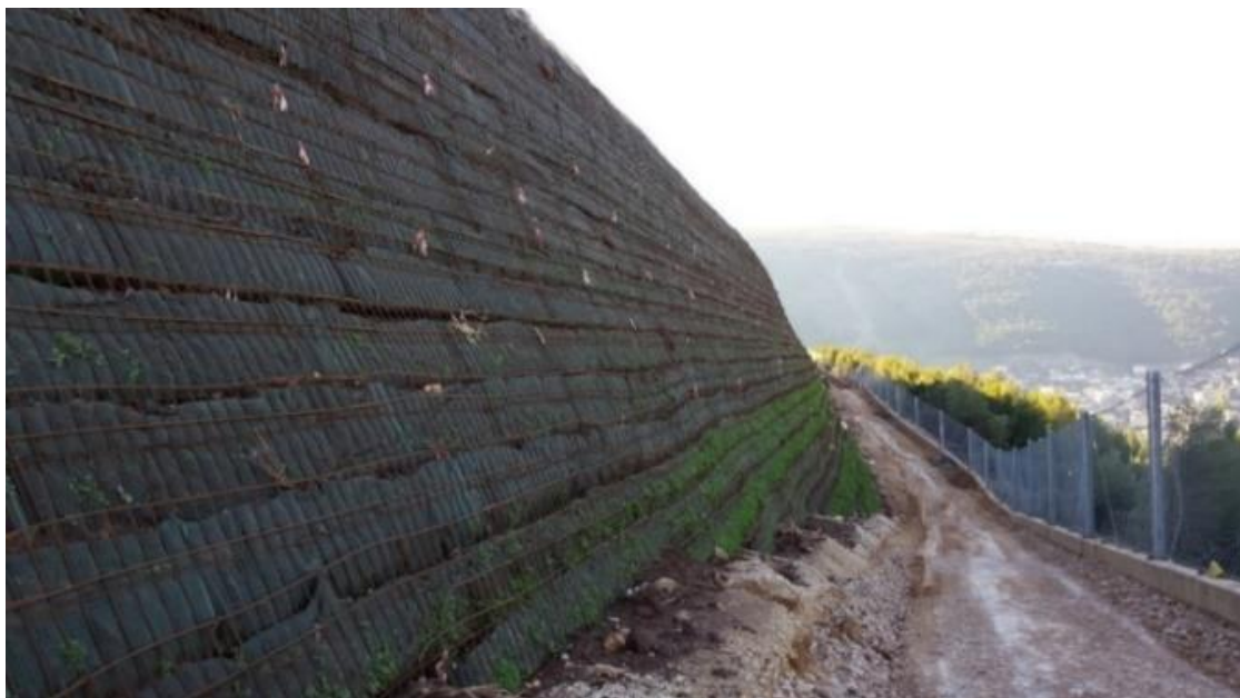
View of reinforced earth fill with wrap-around technique of the reinforcement (Ionian highway)
