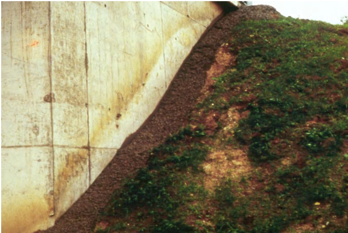
Figure 1. Rainfall induced collapse of a bridge abutment. Note that the embankment settled and deformed horizontally
