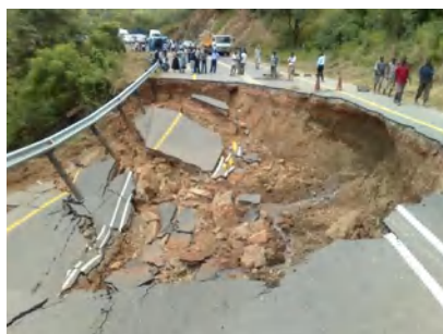
a. Road Failure
