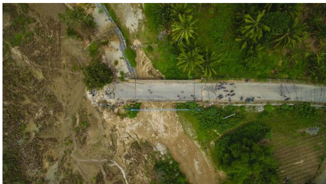
Collapsed bridge after the September 2018 earthquake and tsunami that hit Central Sulawesi. Credit: N.Hariadi
