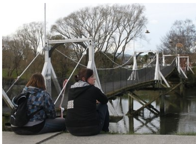
Buckled foot-bridge in Paiapoi, 20km south of Christchurch.
