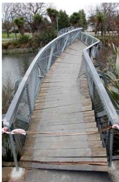
A damaged walking bridge remains over the Avon River in Avonside, Christchurch
