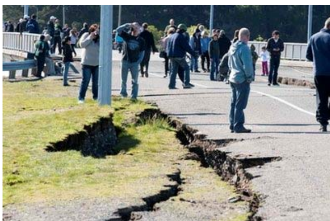
People inspect a crack in the South Brighton Bridge approach in Christchurch.
