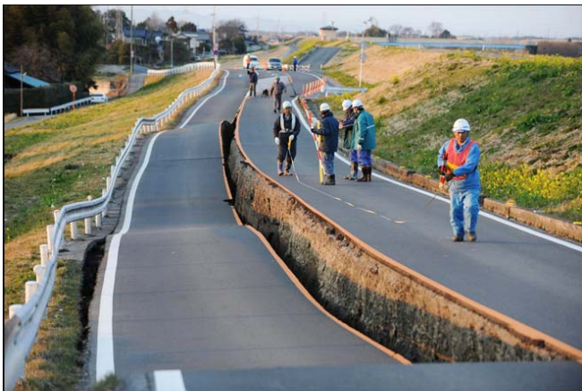
Collapsed section of a road in Saitama Prefecture
